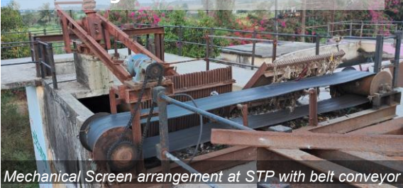
Existing 20 MLD STP treatment
